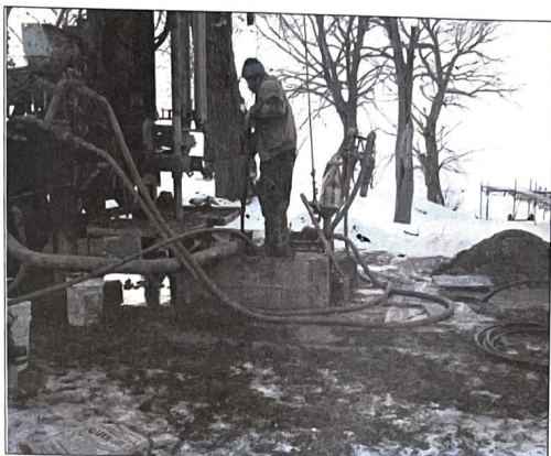
A workman from Advanced Custom Geothermal LLC, located in St. Cloud and Kiel, operates heavy equipment for installation of a geothermal heating and cooling system at the home of Tom Schuppe and his wife, Karen Lindberg-Schuppe, along the East Shore of Lake Winnebago.
